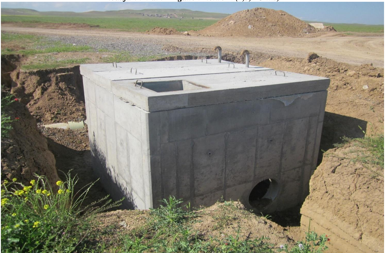
Valves Control Boxes Khodafarin Main Irrigation Network (2,3,4 Units)
