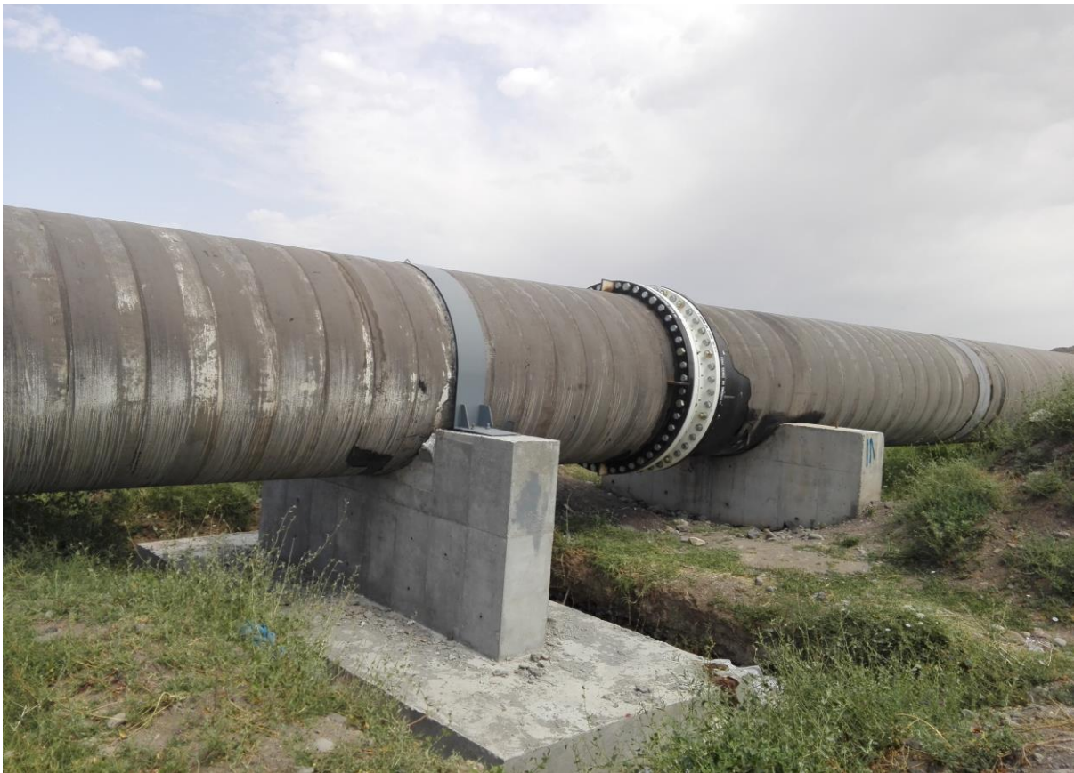
Metal Pipe Syphon Operation Execution of South- North Syphon of Sabalan Dam
