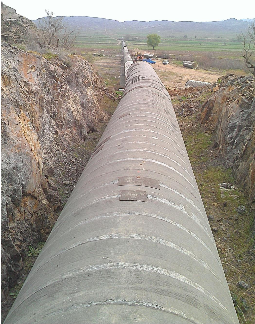
Metal Pipe Siphon Operation Execution of South- North Syphon of Sabalan Dam
