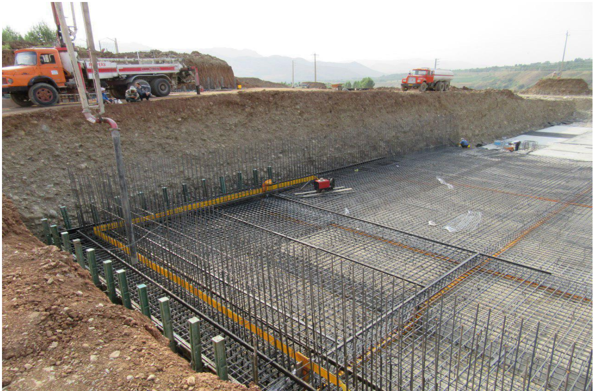
Reservation Pomp Station Execution of Grade 1 Water Supply Pipes of Badin2 Plain
