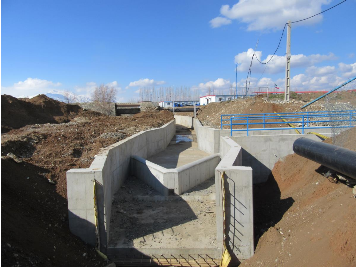
Hydro mechanical Structures Execution of Grade 1 Water Supply Pipes of Badin2 Plain
