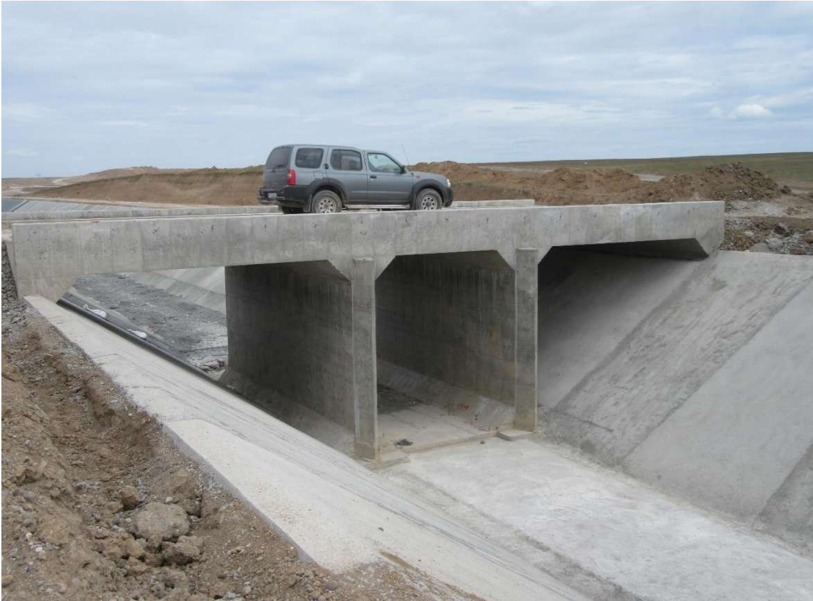
Bridge Khodafarin Irrigation and Drainage Network and Technical Structures 2
