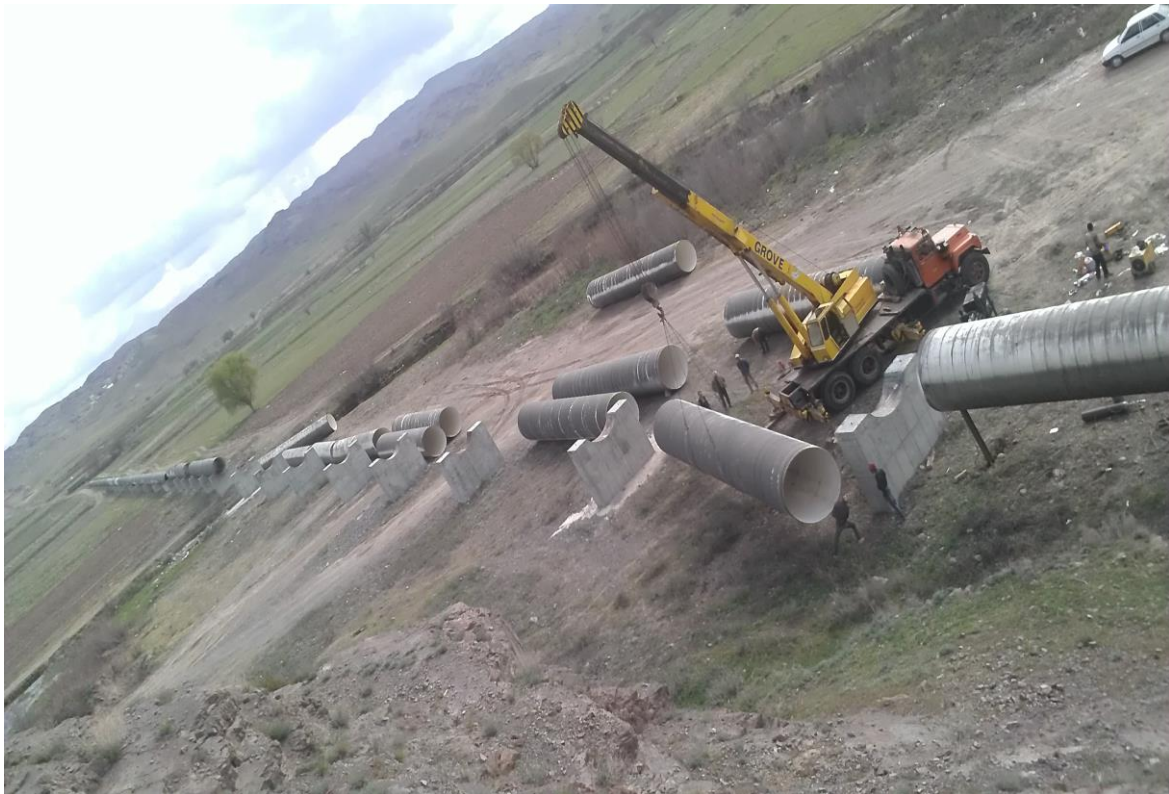
Metal Pipe Syphon Operation Execution of South- North Syphon of Sabalan Dam
