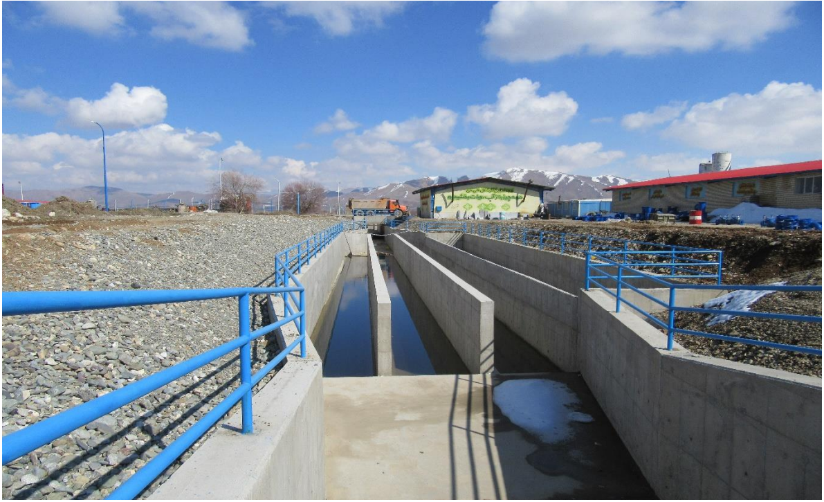
Hydro mechanical Structures Execution of Grade 1 Water Supply Pipes of Badin2 Plain
