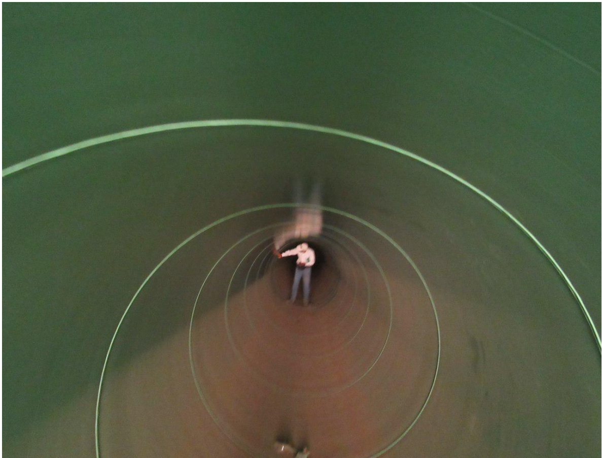
Epoxy inside Covering Execution of Grade 1 Water Supply Pipes of Badin 2 Plain
