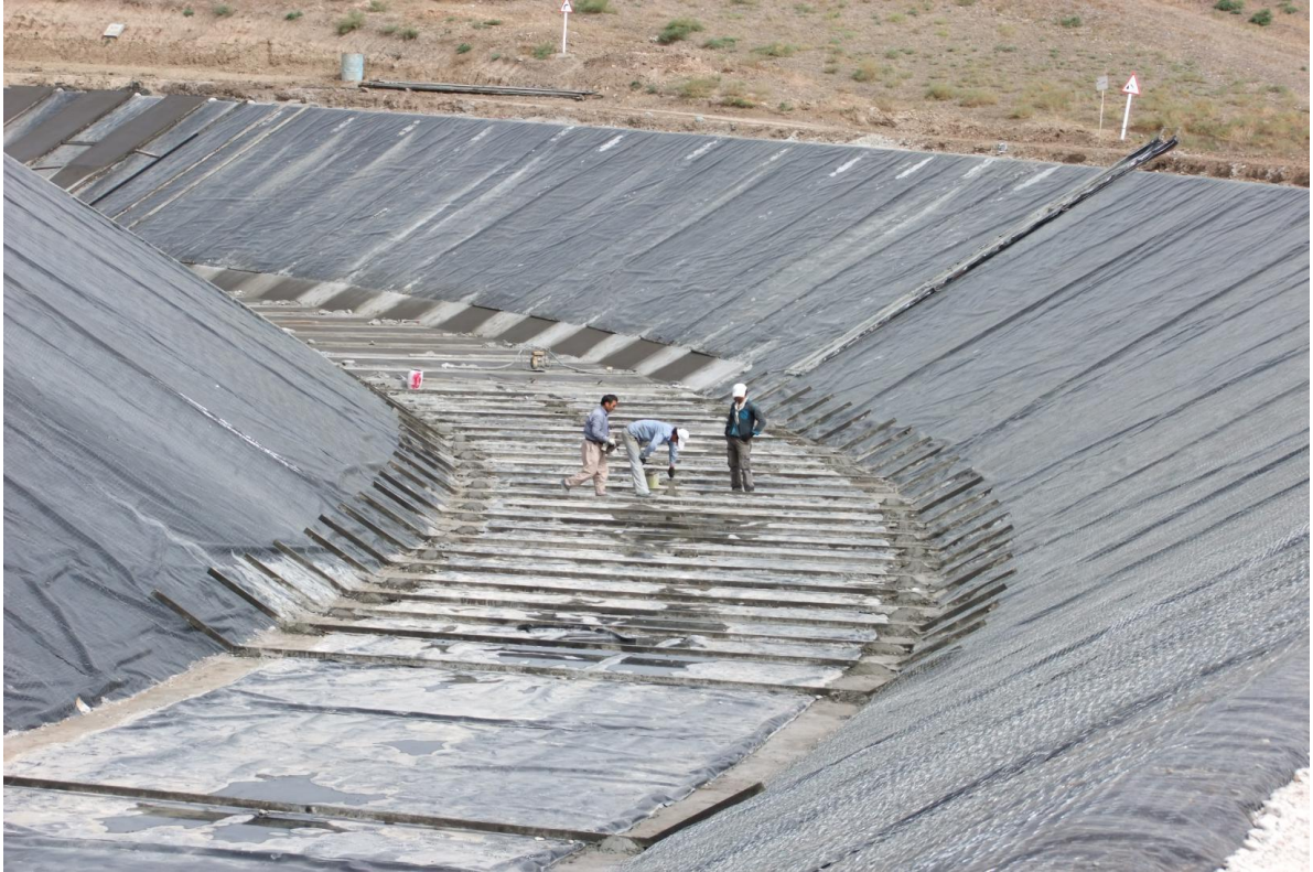
Geomamberian Khodafarin Irrigation and Drainage Network and Technical Structures 2
