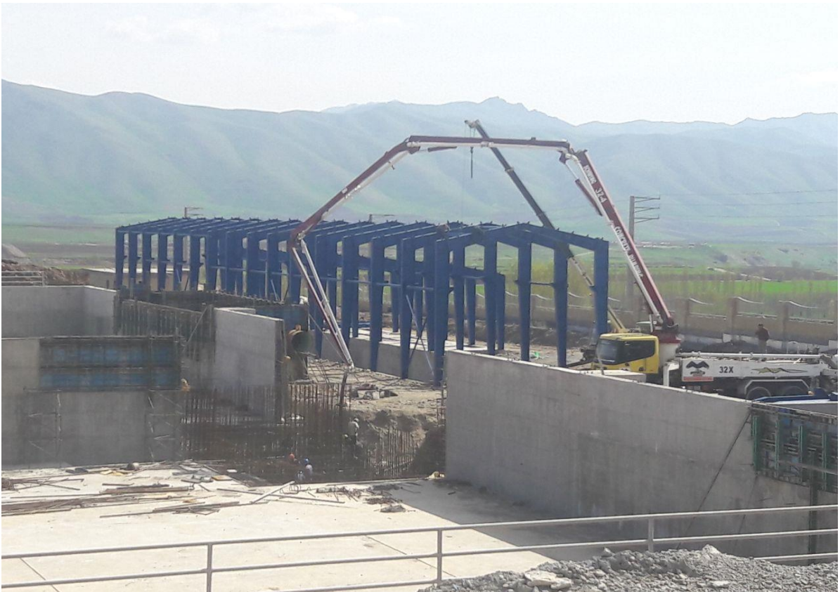
Reservation Structure of Pomp Station Execution of Grade 1 Water Supply Pipes of Badin2 Plain
