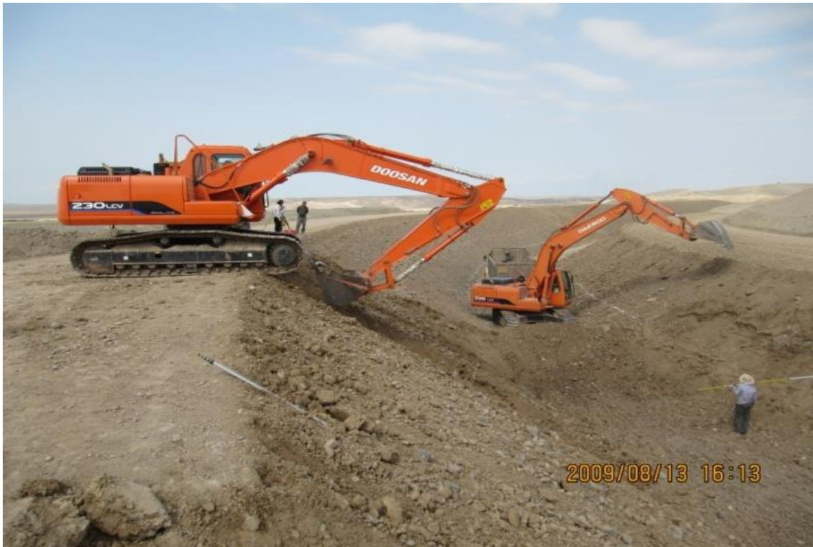
Trimming Khodafarin Irrigation and Drainage Network and Technical Structures 2
