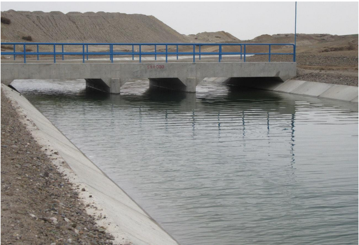
Bridge Khodafarin Irrigation and Drainage Network and Technical Structures 2
