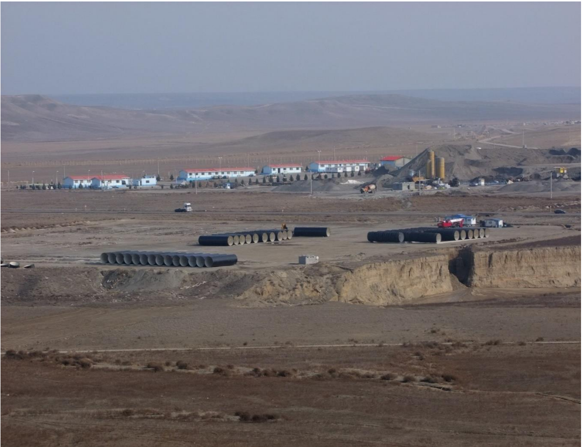
Mobilization, Offices & Workshop Khodafarin Irrigation and Drainage Network and Technical Structures project
