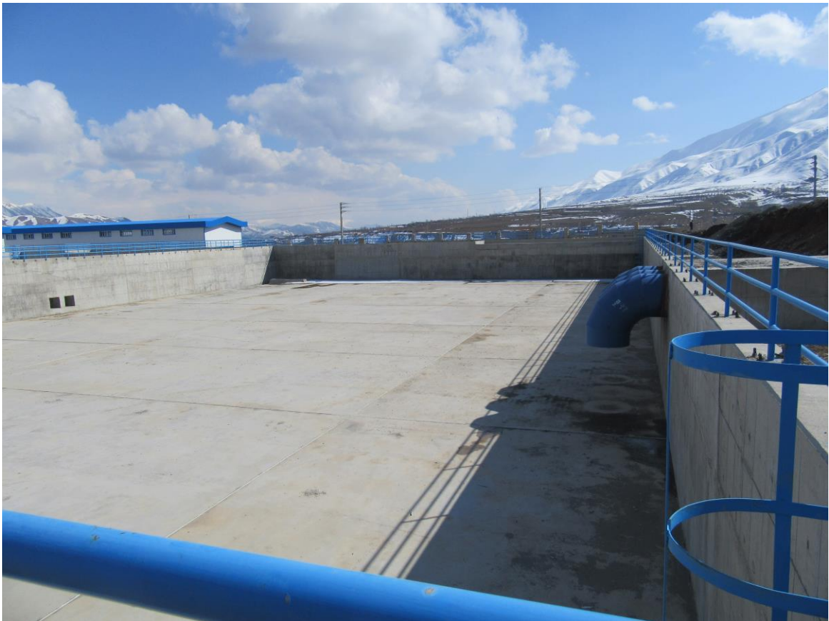
Reservation Structure of Pomp Station Execution of Grade 1 Water Supply Pipes of Badin2 Plain
