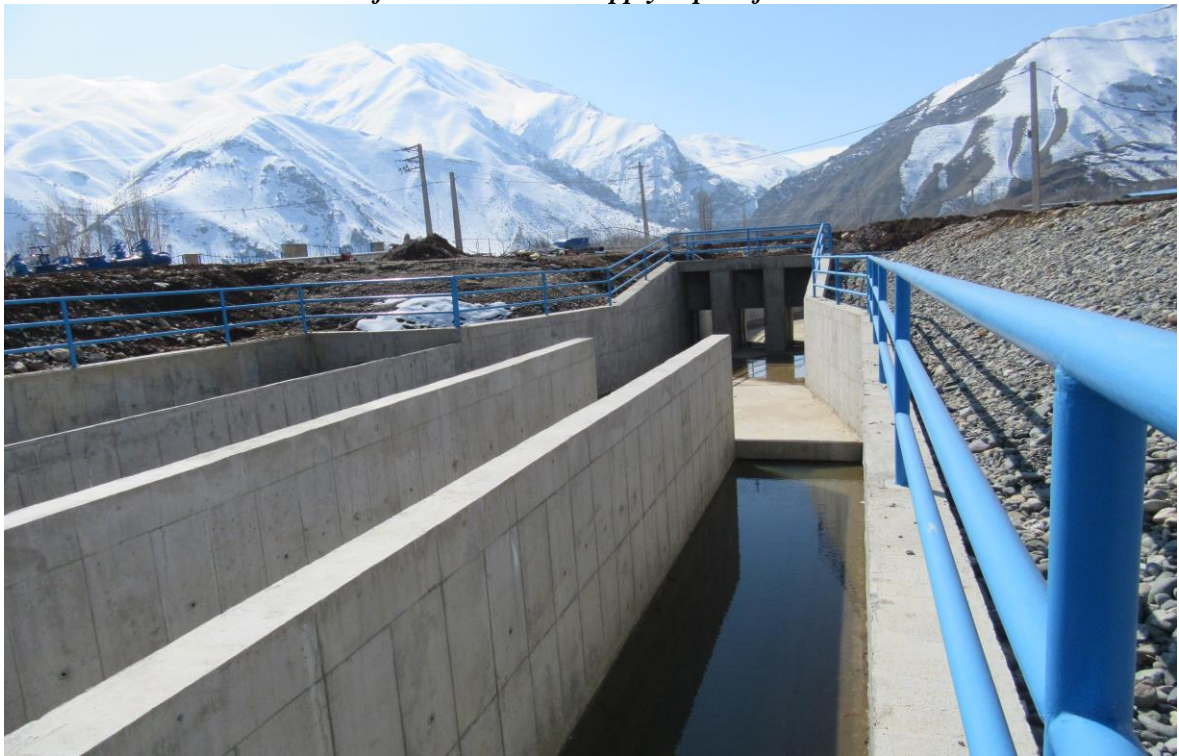
Hydro mechanical Structures Execution of Grade 1 Water Supply Pipes of Badin2 Plain
