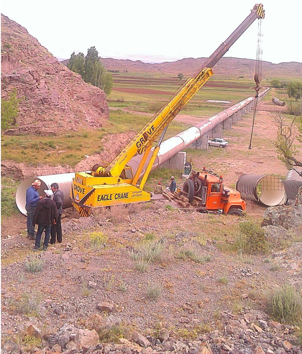
Metal Pipe Syphon Operation Execution of South- North Syphon of Sabalan Dam
