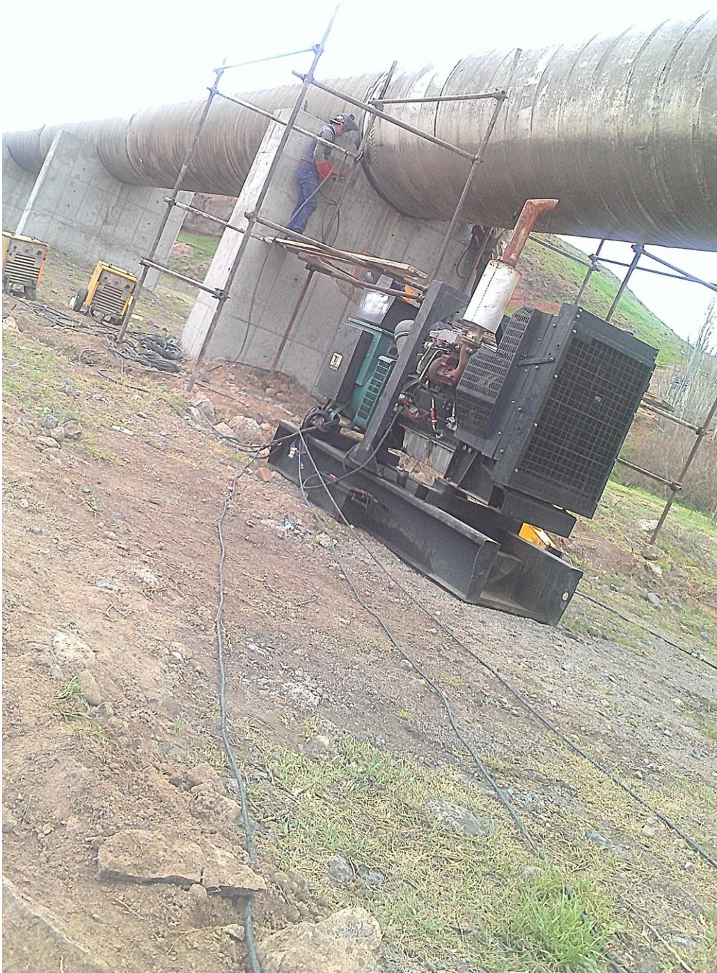
Metal Pipe Syphon Operation Execution of South- North Syphon of Sabalan Dam
