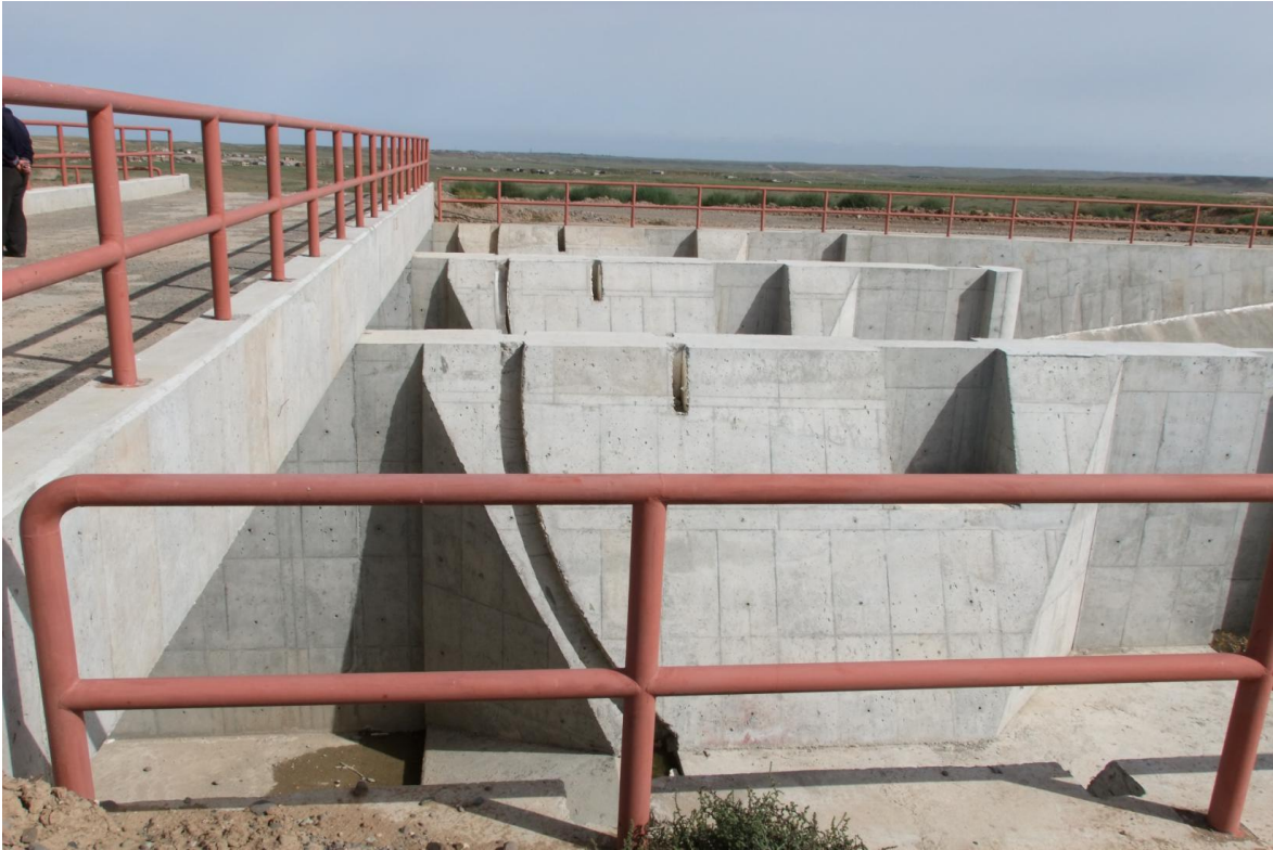
Hydro mechanical Structure Khodafarin Irrigation and Drainage Network and Technical Structures project
