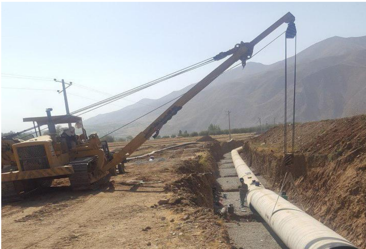
Metal Pipe Syphon Operation Execution of Grade 1 Water Supply Pipes of Badin2 Plain
