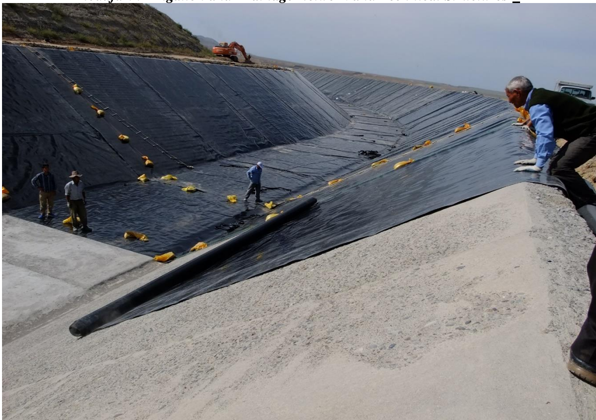
Geomamberian Khodafarin Irrigation and Drainage Network and Technical Structures 2
