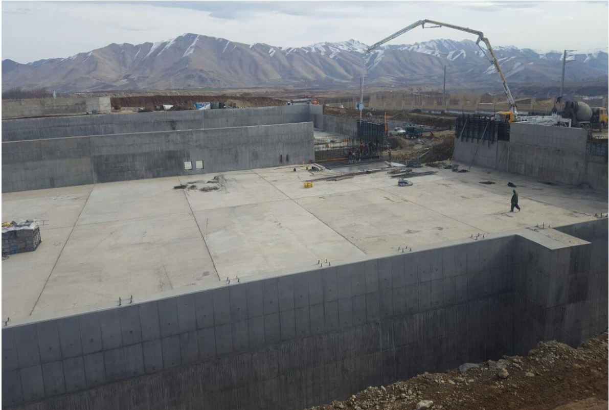
Reservation Structure of Pomp Station Execution of Grade 1 Water Supply Pipes of Badin2 Plain
