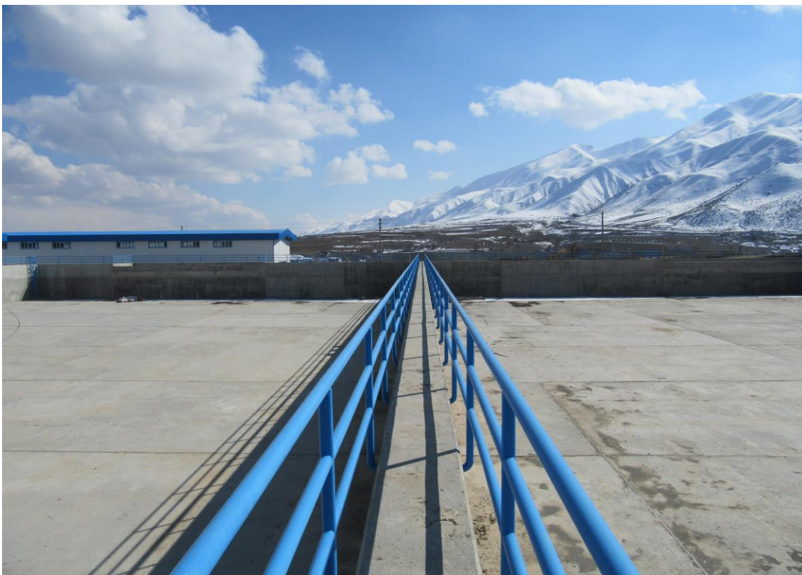
Reservation Structure of Pomp Station Execution of Grade 1 Water Supply Pipes of Badin2 Plain
