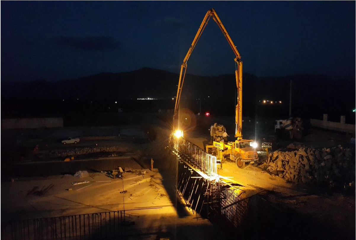
Reservation Pomp Station Execution of Grade 1 Water Supply Pipes of Badin2 Plain
