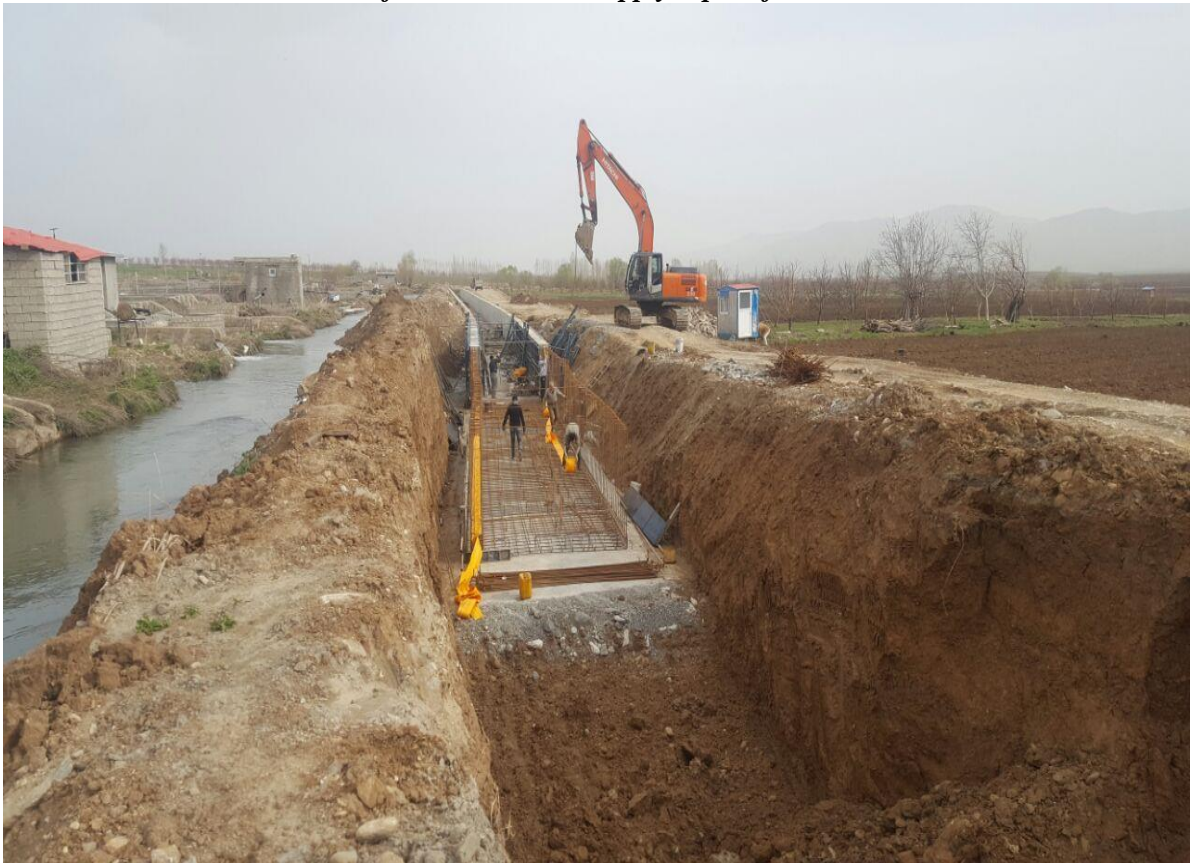
Hydro Mechanical Structures Execution of Grade 1 Water Supply Pipes of Badin1 Plain
