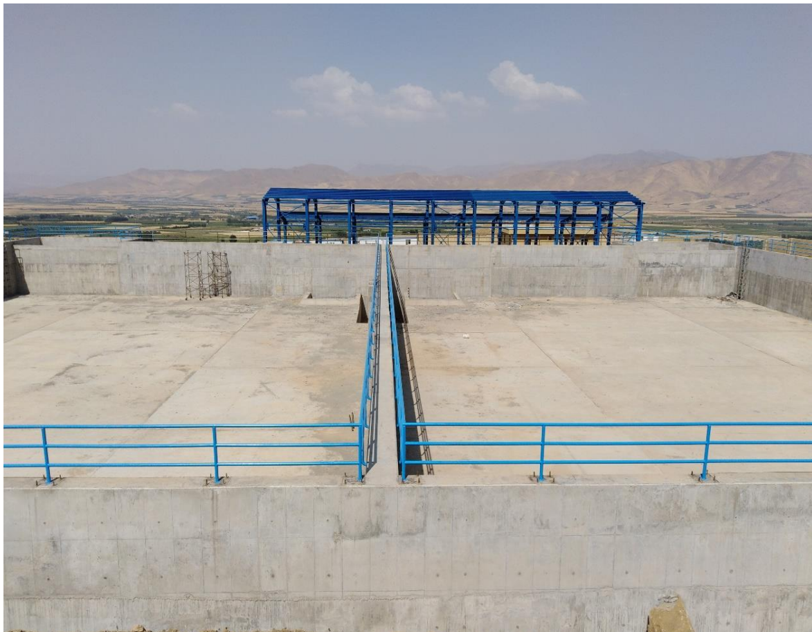
Reservation Structure of Pomp Station Execution of Grade 1 Water Supply Pipes of Badin2 Plain
