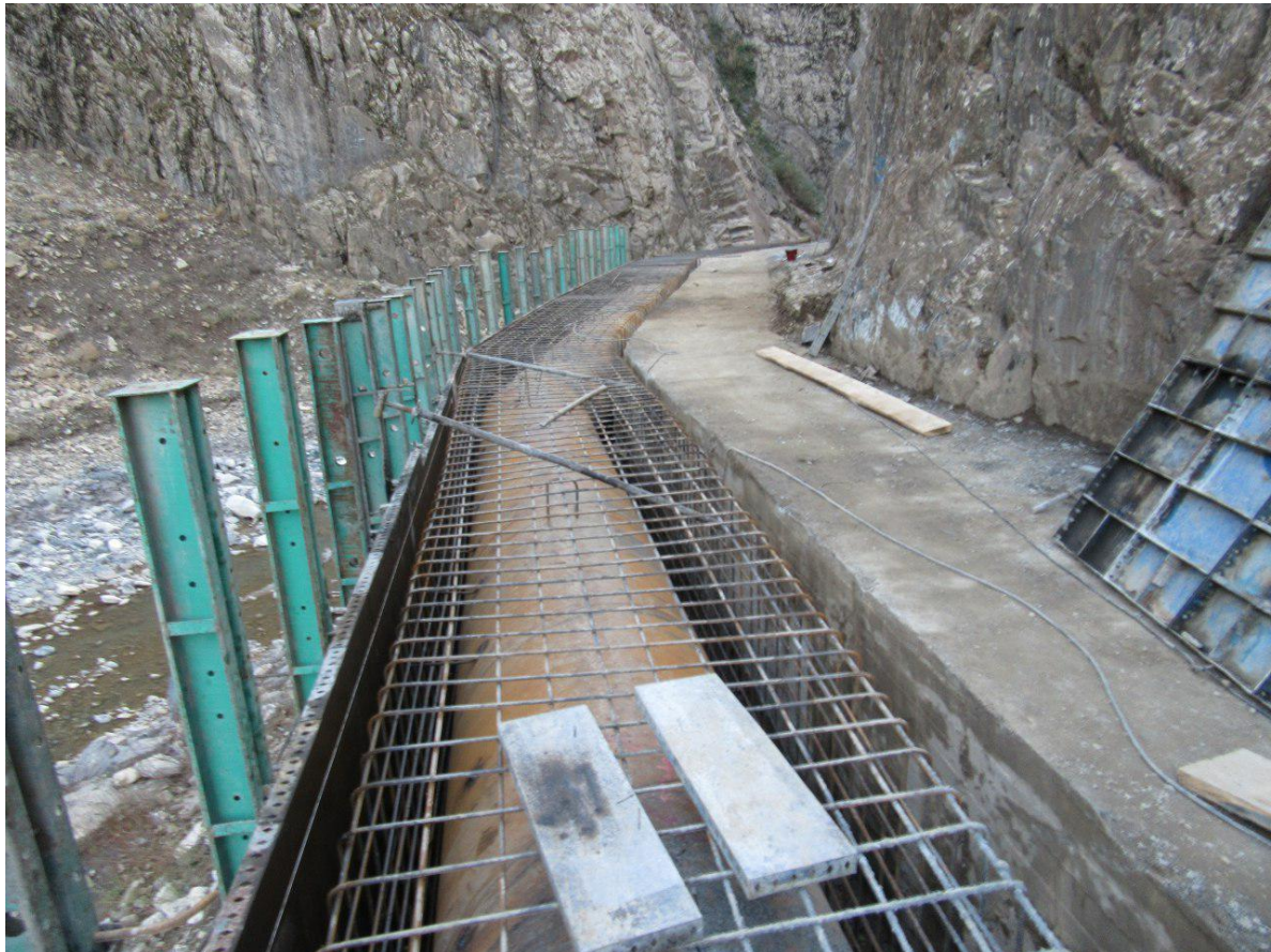
Metal Pipe Syphon Operation Execution of Grade 1 Water Supply Pipes of Badin2 Plain
