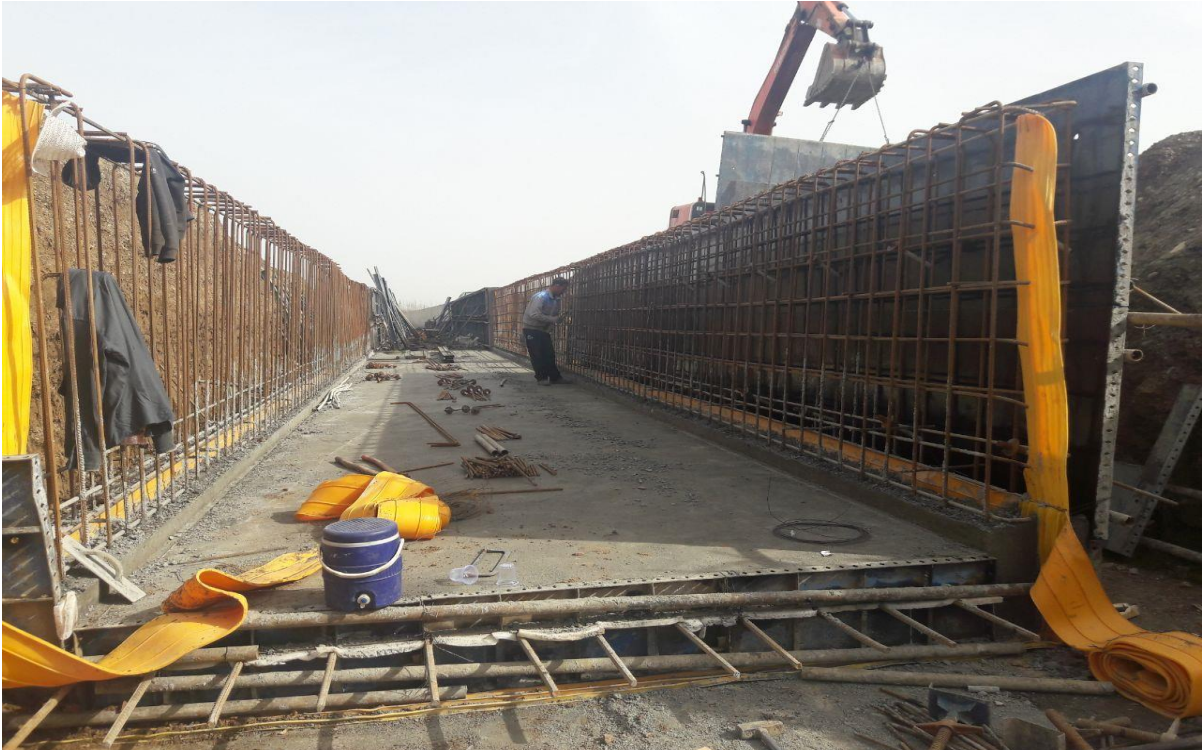
Hydro Mechanical Structures Execution of Grade 1 Water Supply Pipes of Badin1 Plain
