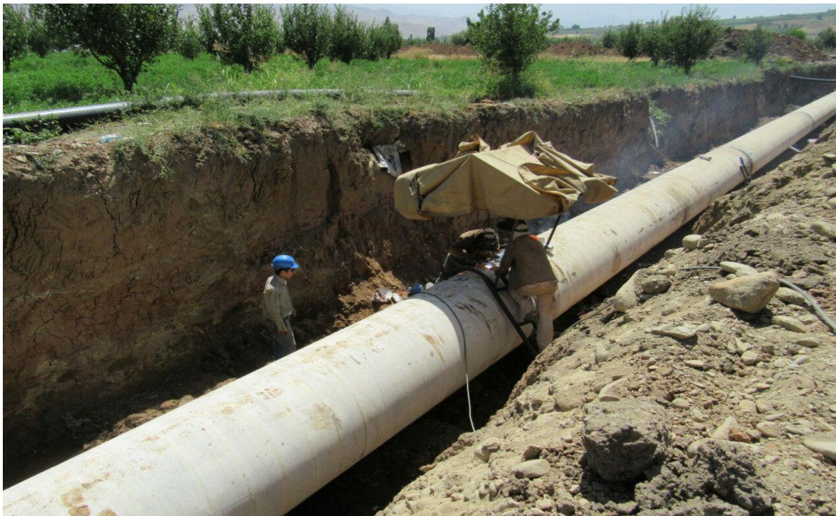
Metal Pipe Syphon Operation Execution of Grade 1 Water Supply Pipes of Badin2 Plain
