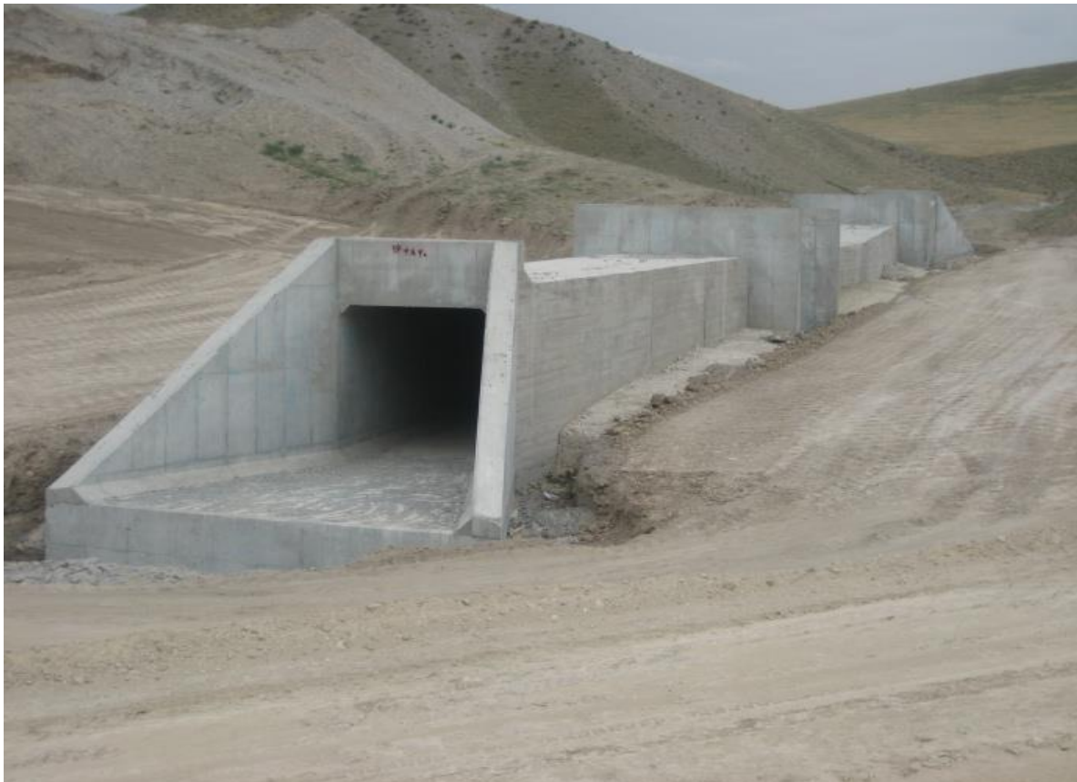
Hydro mechanical Structure Khodafarin Irrigation and Drainage Network and Technical Structures project
