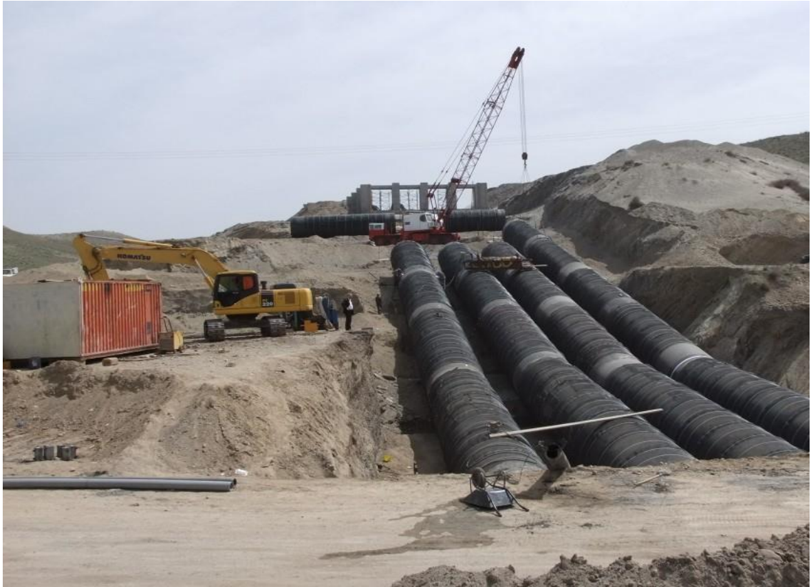
Metal Pipe Syphon Operation Khodafarin Irrigation and Drainage Network and Technical Structures project
