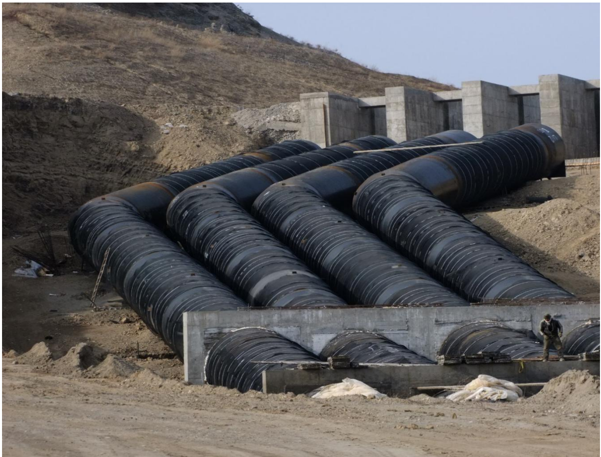
Metal Pipe Syphon Operation Khodafarin Irrigation and Drainage Network and Technical Structures project
